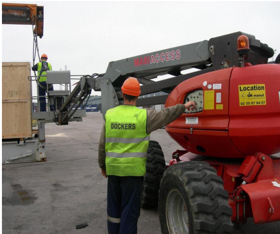
Figure 48 Use of MEWP (Mobile Elevating Work Platform). Note protection of worker in cage.
