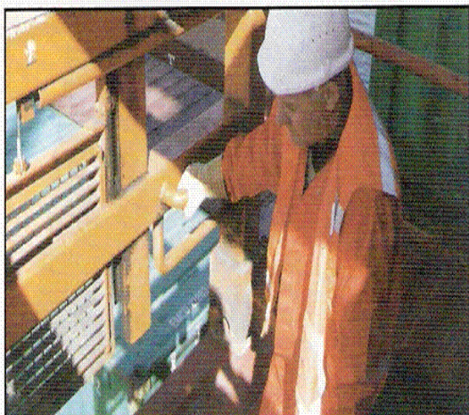
Figure 24 Recessed handrails inside personnel cage
