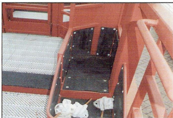
Figure 33 Bins for container securing equipment. Note recessed hand rail and raised end floor
