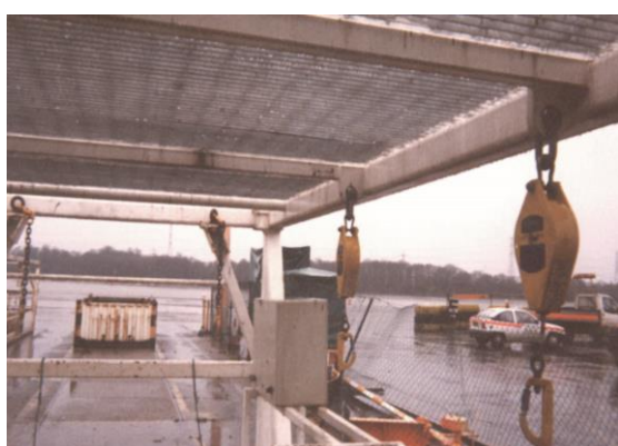
Figure 104 Fall arrest block anchorage to eyes at the top of a personnel cage.
