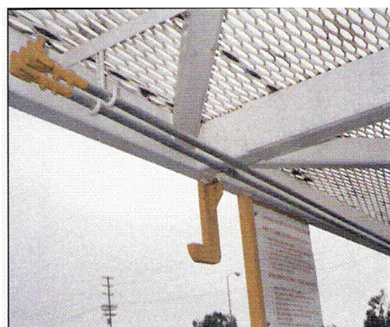
Figure 36 Hooks on roof for twistlock poles or rescue hooks. Note roof covering.
