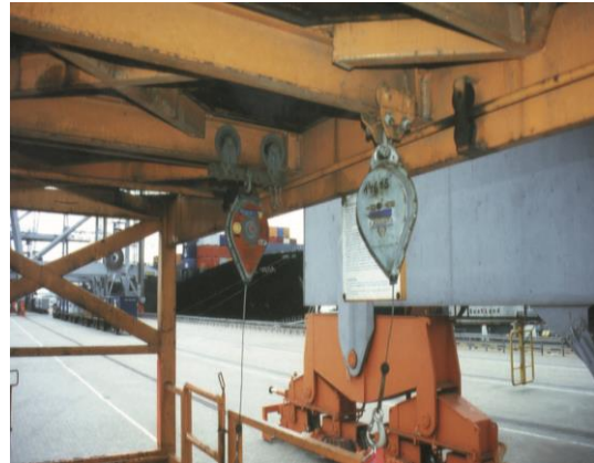
Figure 107 Personnel cage including four fall arrest blocks on runway beams
