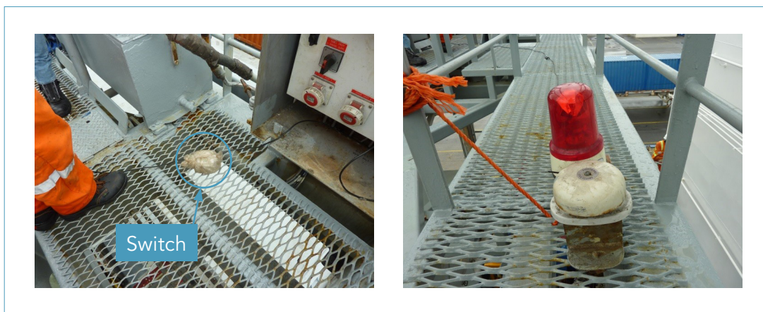
Alternative alarm system with on the left (figure 8) the switch and on the right (figure 9) the alarm bell and the strobe light.
