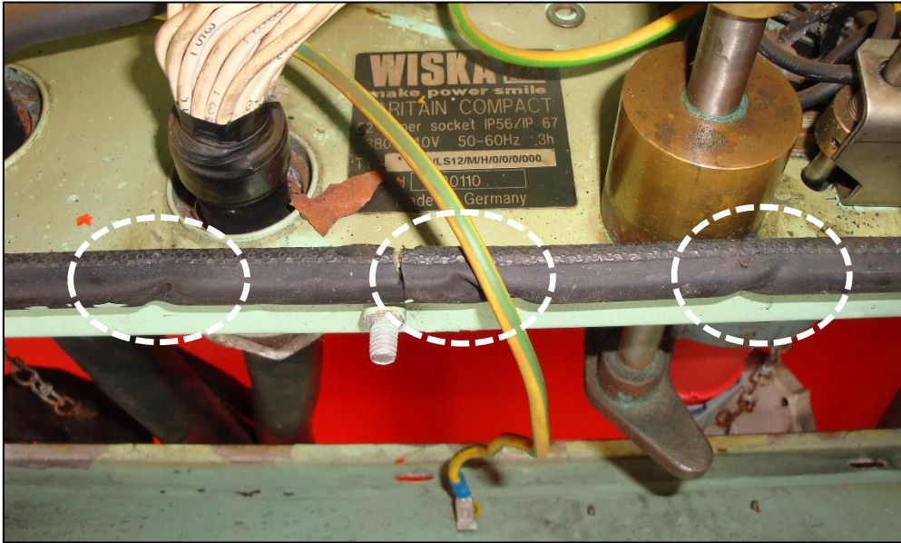
Figure 2: Localized pressure points in the rubber seal of the switch box housing
