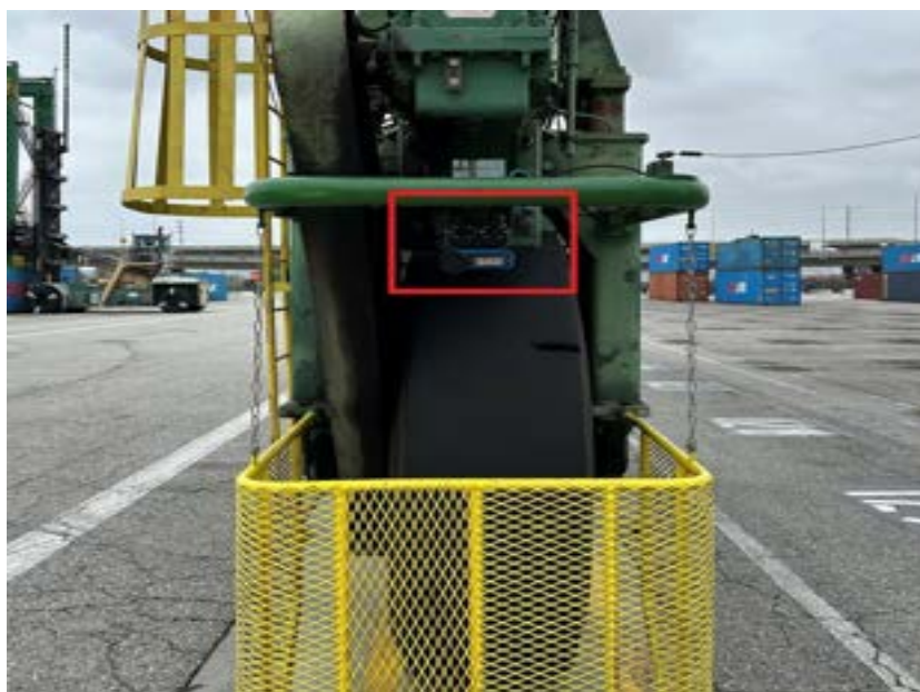
Location of cameras on RTG
